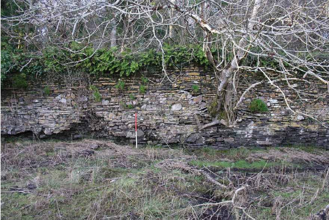
Photo 35: Closer view of the southern wall of the garden enclosure, viewed from the south. 1m scale.
