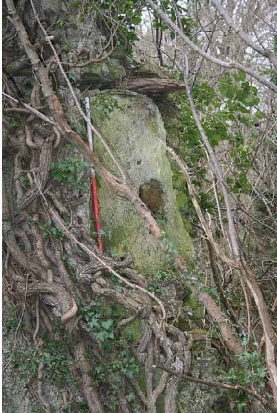
Photo 25: 1 st floor window remains in the southern wall of the Western Tower, also showing surviving timber lintel. 1m scale.
