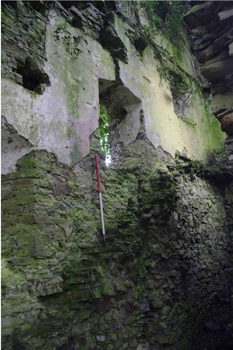
Photo 11: Interior of Eastern Tower showing staircase remains and internal render. 1m scale
