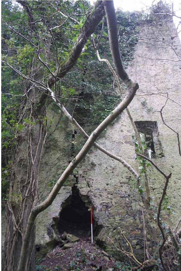
Photo 9: Closer view of the collapsed archway and vertical crack above. 1m scale.
