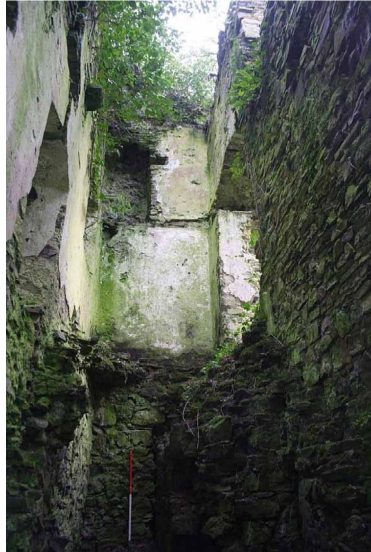
Photo 12: Interior of Eastern Tower showing different floor levels and 3 rd floor fireplace. 1m scale.
