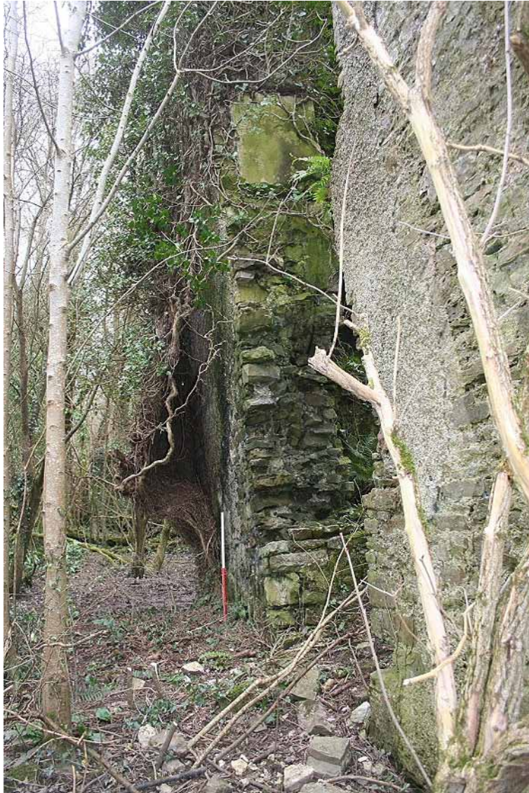
Photo 17: Looking north along the western wall of the Western Tower, showing the outward lean. 1m scale.
