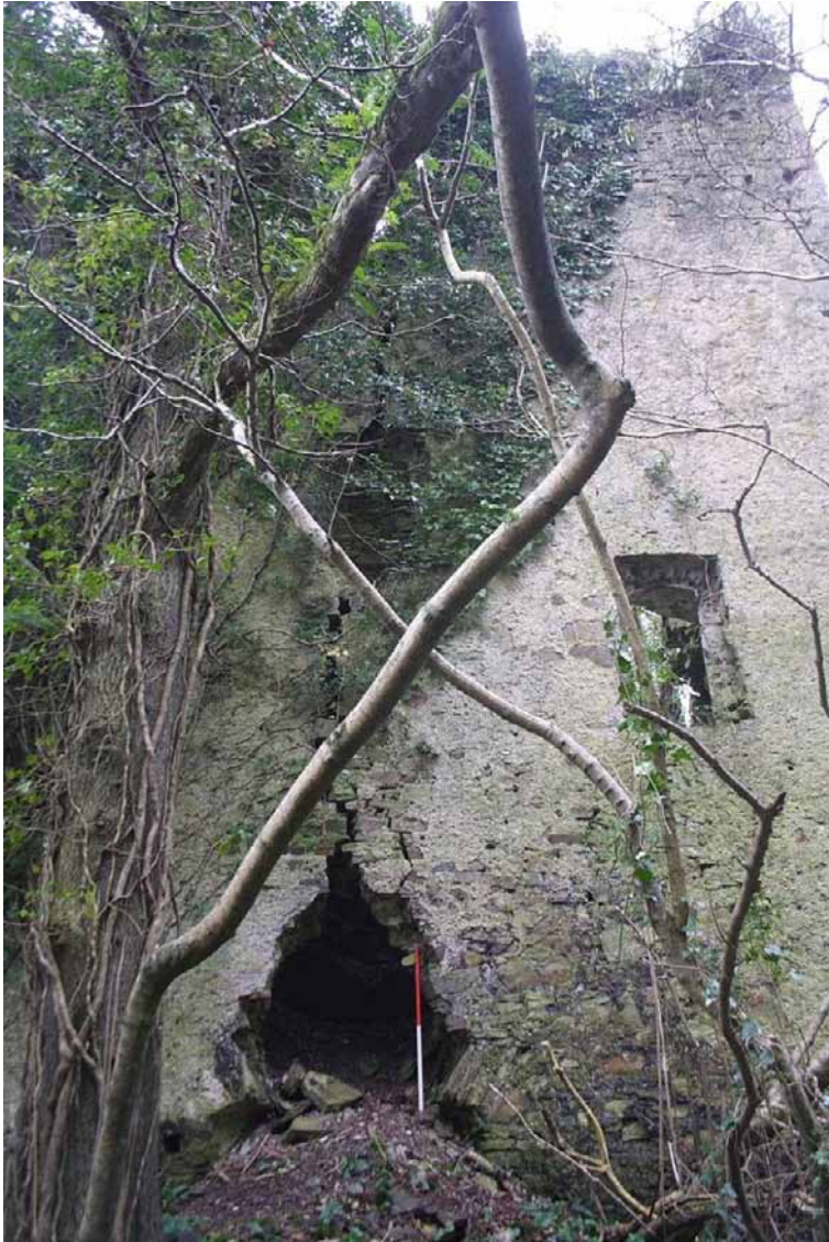
Photo 9: Closer view of the collapsed archway and vertical crack above. 1m scale.
