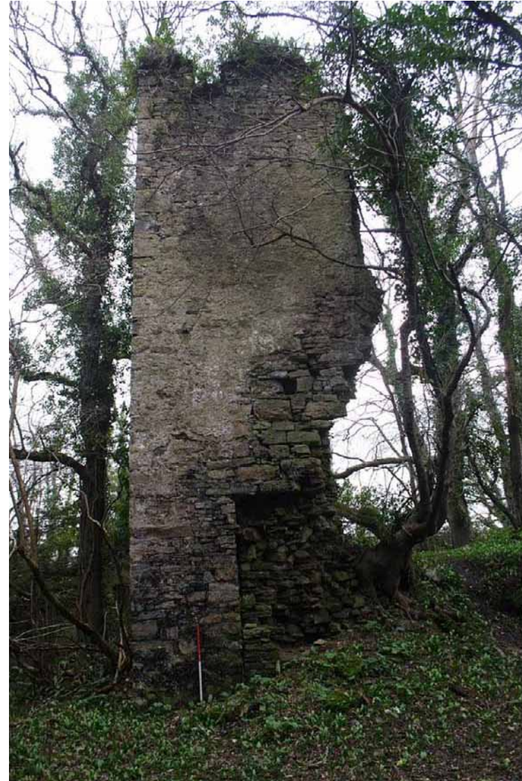
Photo 10: Northern face of Eastern Tower, clearly showing earlier segment of walling. 1m scale.
