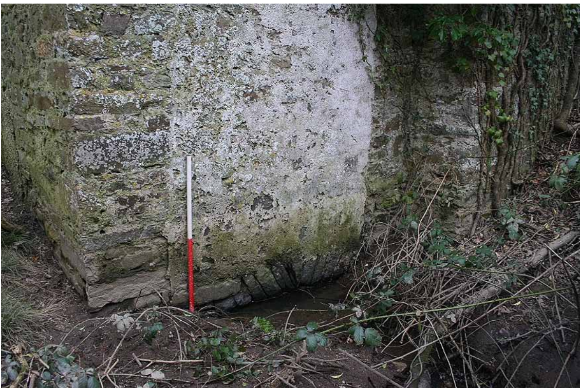
Photo 22: Stream emerging from the culvert on the south side of the Western Tower. 1m scale.
