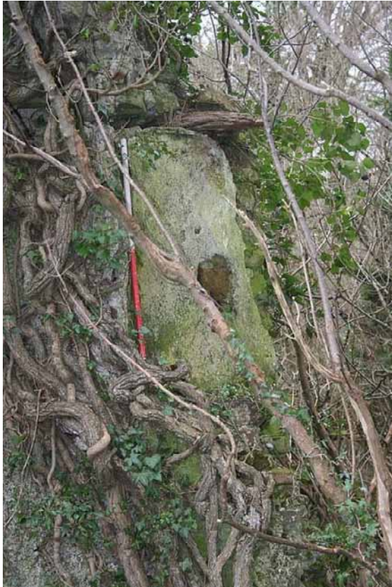
Photo 25: 1 st floor window remains in the southern wall of the Western Tower, also showing surviving timber lintel. 1m scale.
