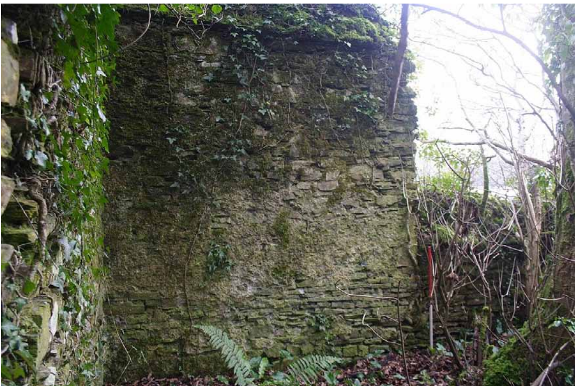
Photo 42: Interior of the southern wall at the southeast corner of the Garden Enclosure. Straight vertical joint visible to the left of the 1m scale.
