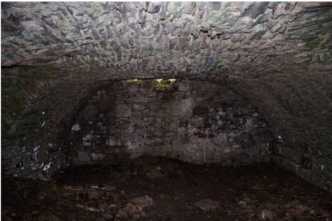
Photo 32: The interior of the undercroft looking west, showing the collapse in the ceiling and upper courses of the western wall. 1m scale.
