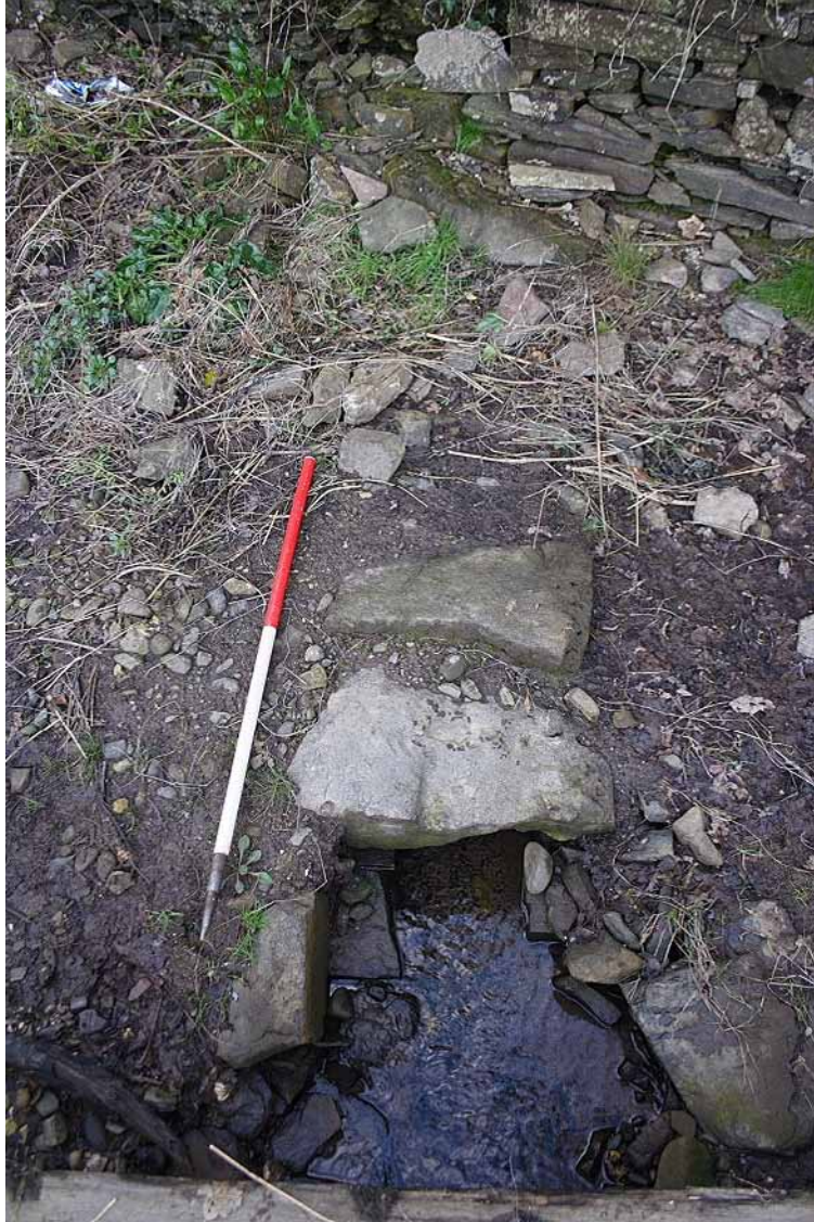
Photo 53: Culverted stream running out from underneath the Southwest Enclosure, looking north. 1m scale.
