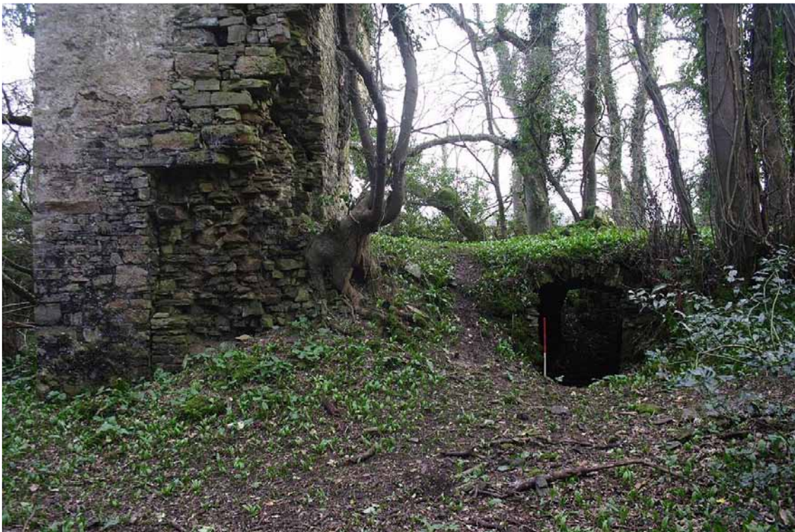
Photo 26: View south towards the Eastern Tower and main entrance into the undercroft. 1m scale.
