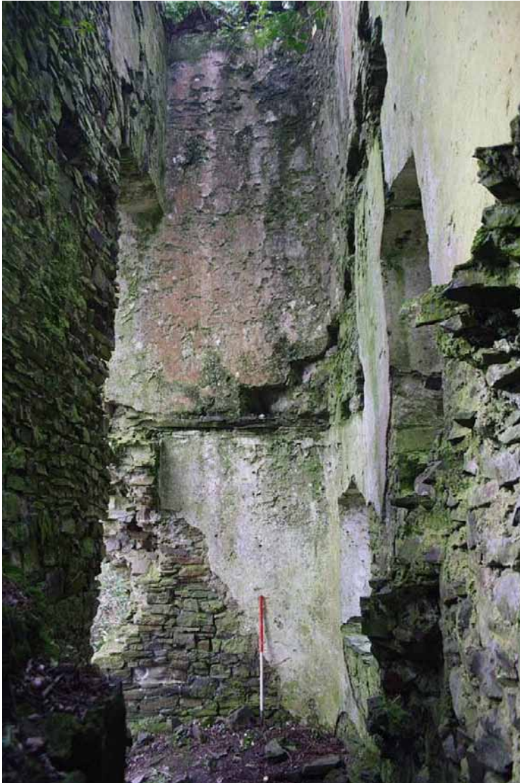
Photo 13: Interior of Eastern Tower showing pinker internal render on 2 nd floor. 1m scale.
