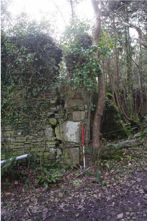
Photo 43: Damage at the north-eastern corner of the Garden Enclosure. 1m scale.
