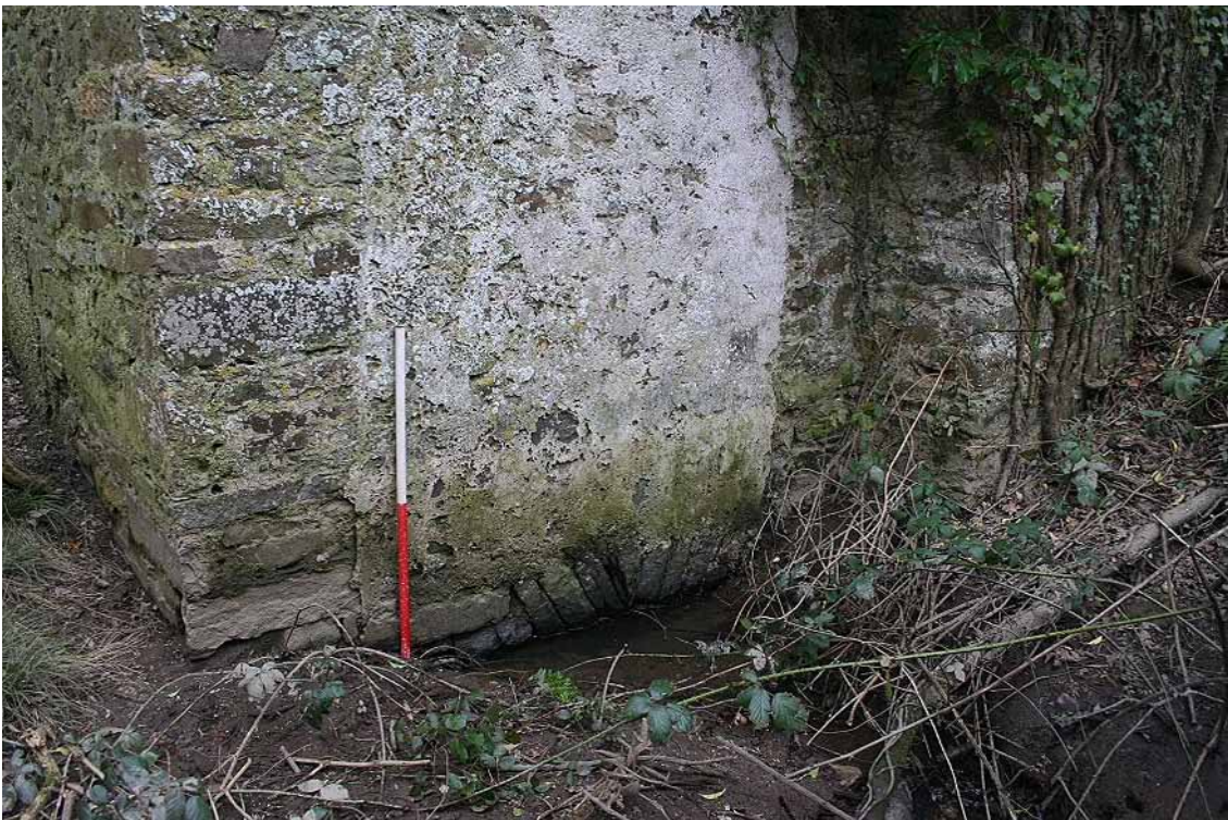
Photo 22: Stream emerging from the culvert on the south side of the Western Tower. 1m scale.
