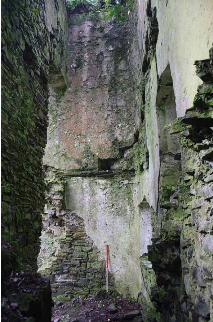
Photo 13: Interior of Eastern Tower showing pinker internal render on 2 nd floor. 1m scale.
