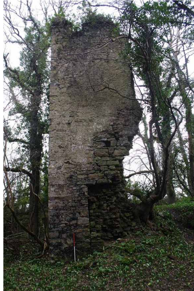
Photo 10: Northern face of Eastern Tower, clearly showing earlier segment of walling. 1m scale.
