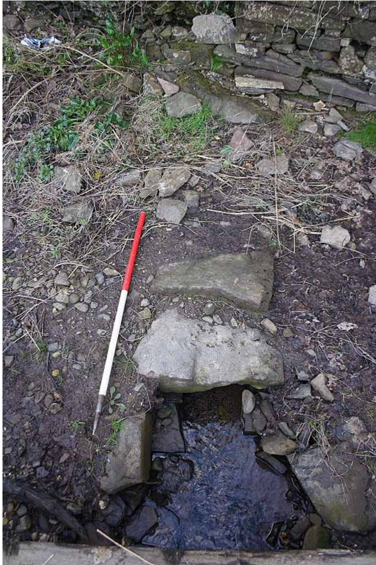
Photo 53: Culverted stream running out from underneath the Southwest Enclosure, looking north. 1m scale.
