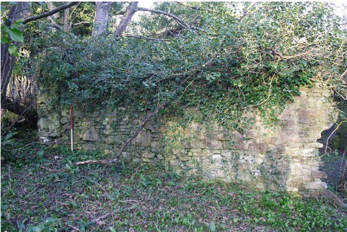
Photo 46: View looking east at the eastern wall of the Southwest Enclosure. 1m scale.
