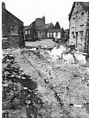
17. Foundation trench for new boundary wall, looking east toward the Market Square
