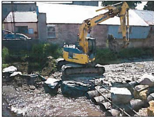
Plate 3. Dredging of river in area of Tregaron bridge. Looking east from bridge.
