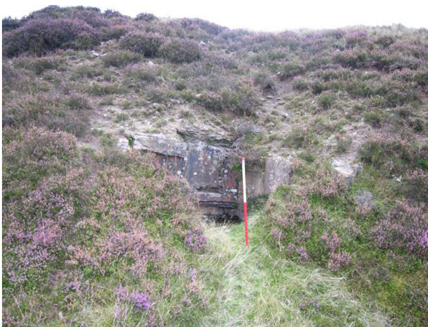
Plate 48. Adit/level portal EA042.09.47 partially blocked, view to east
