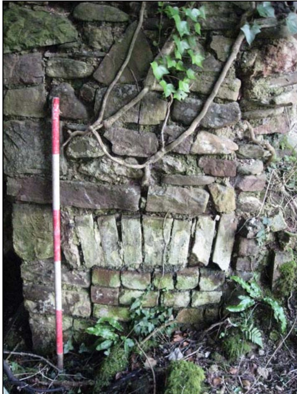
Plate 69: View of a blocked door or window at Caerwigae Mill (PRN 03975s). View to W.
