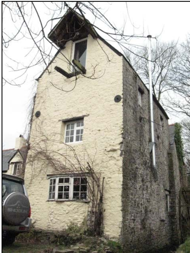
Plate 27: View of the SE facing elevation of Llanfythyn Mill (PRN 01993s). View to NW.
