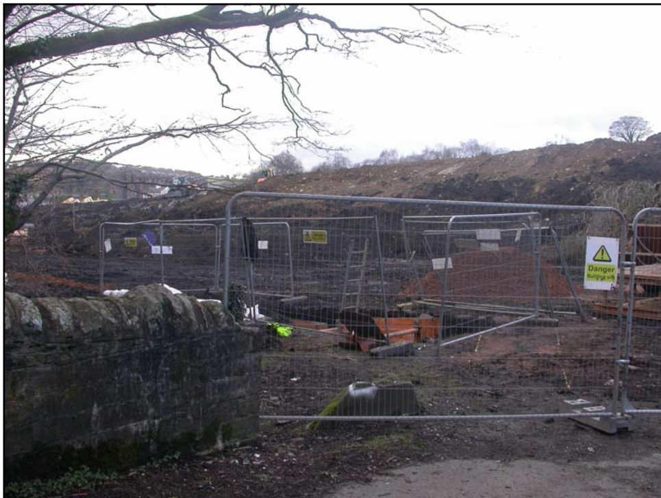
Plate 6: View of construction site from the footbridge at location for Melin Cylla Mill (PRN 00663m). View to NW.
