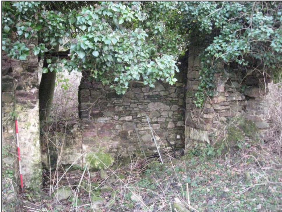
Plate 66: General view of Caerwigae Mill (PRN 03975s) with a blocked doorway. View to S.
