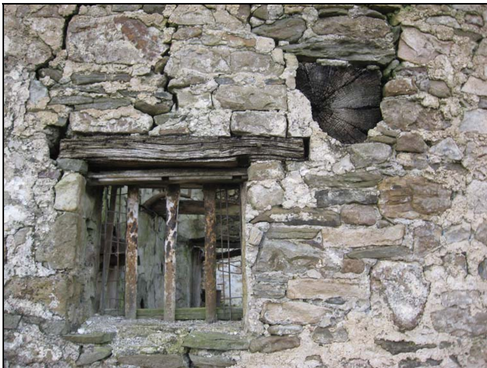
Plate 110: Detail of window and timber lintel on SE elevation of Machen Mill (MP027). View to NW.
