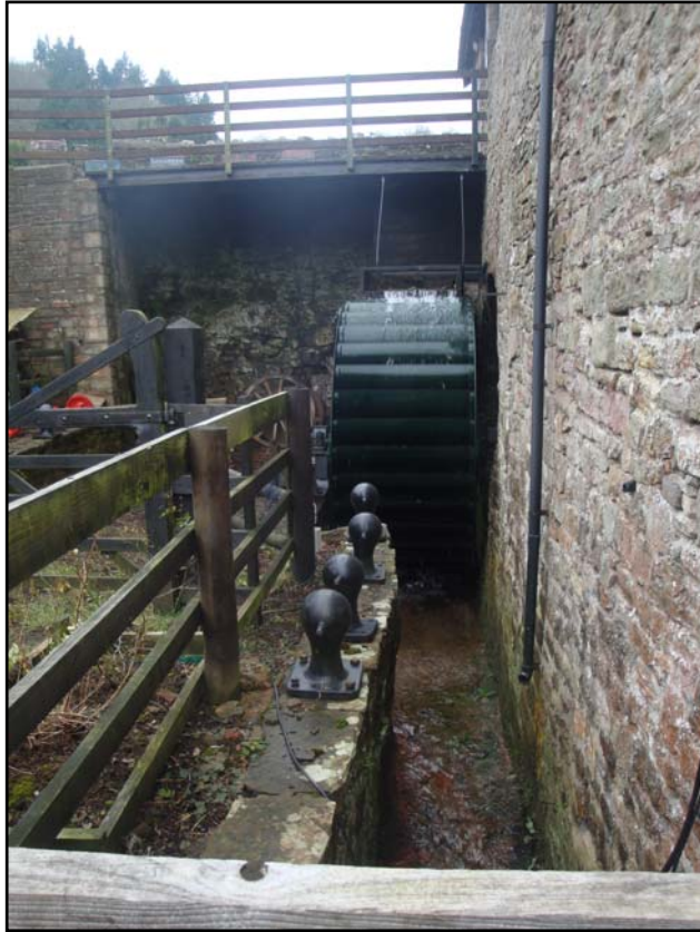
Plate 85: View of the wheel and wheel pit on the SE side of the mill at the Water Wheel (PRN 05687g). View to SW.
