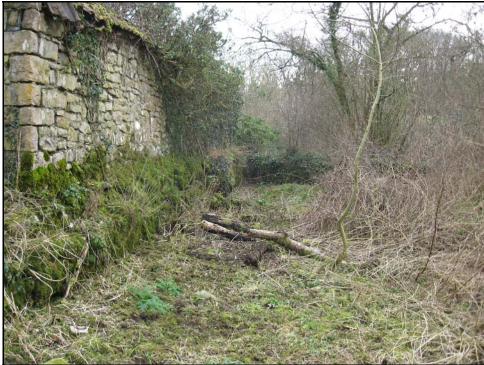
Plate 3: View of Mill race to NW of corn mill (PRN 00283s), near Llanmihangel. View to S.
