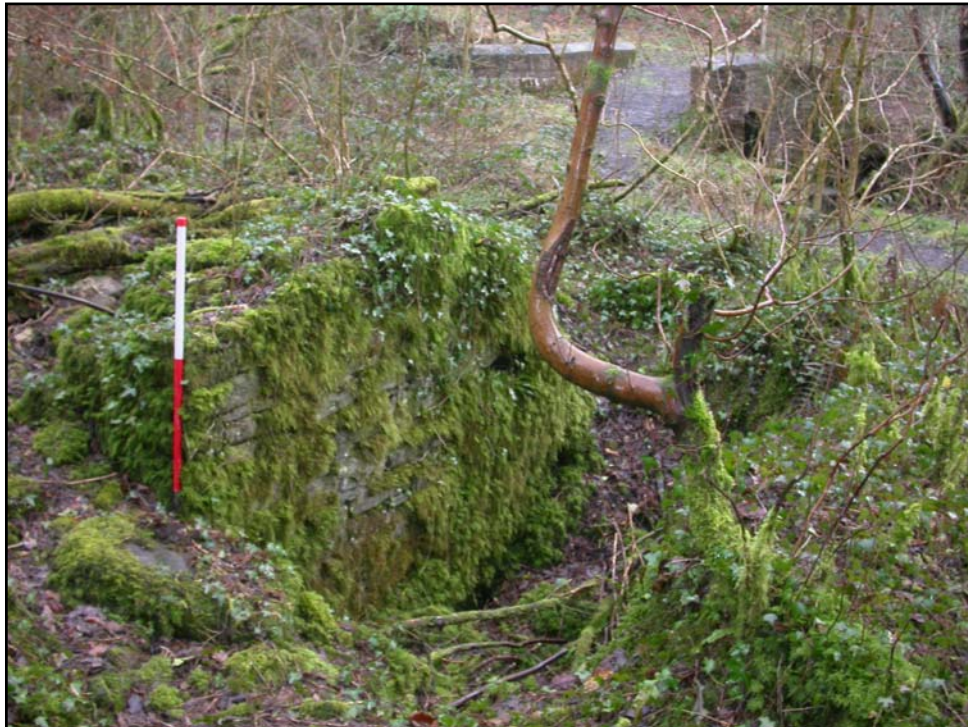
Plate 104: Eastern end of wheel pit at Melin Gelligron Mill (MP020), Pontardawe, with the bridge adjacent to the mill in the background. View to NE.
